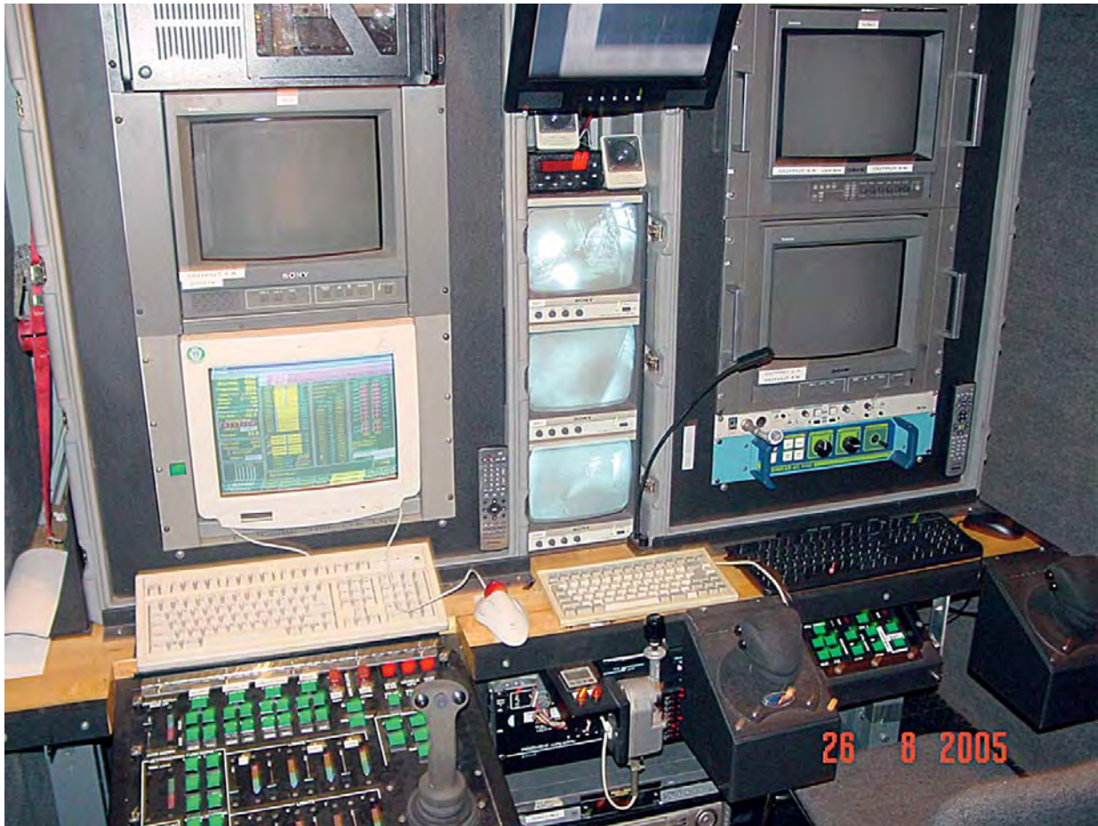
Photo 46: Remora 6000 control room.
